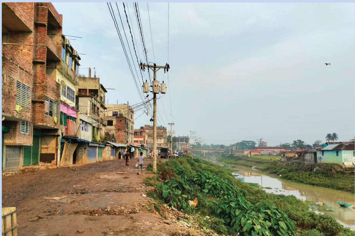
Figure – 8 : Construction of walkway at the left bank of Sonai river after the encroached structures.
